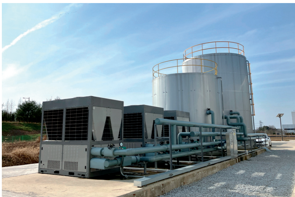
Fig. 4. Installed dual-tank air-source heat pump system at the test greenhouse.
